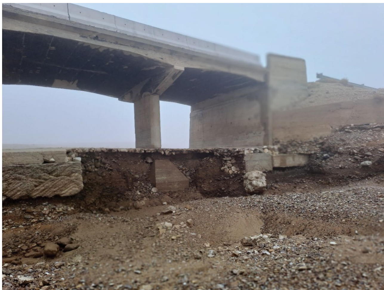
Figure 7: Flood damage Maan area in 2023.
