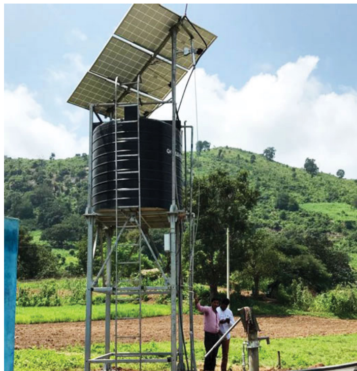
Figure 14: Built PV irrigation system with water reservoir [22].
